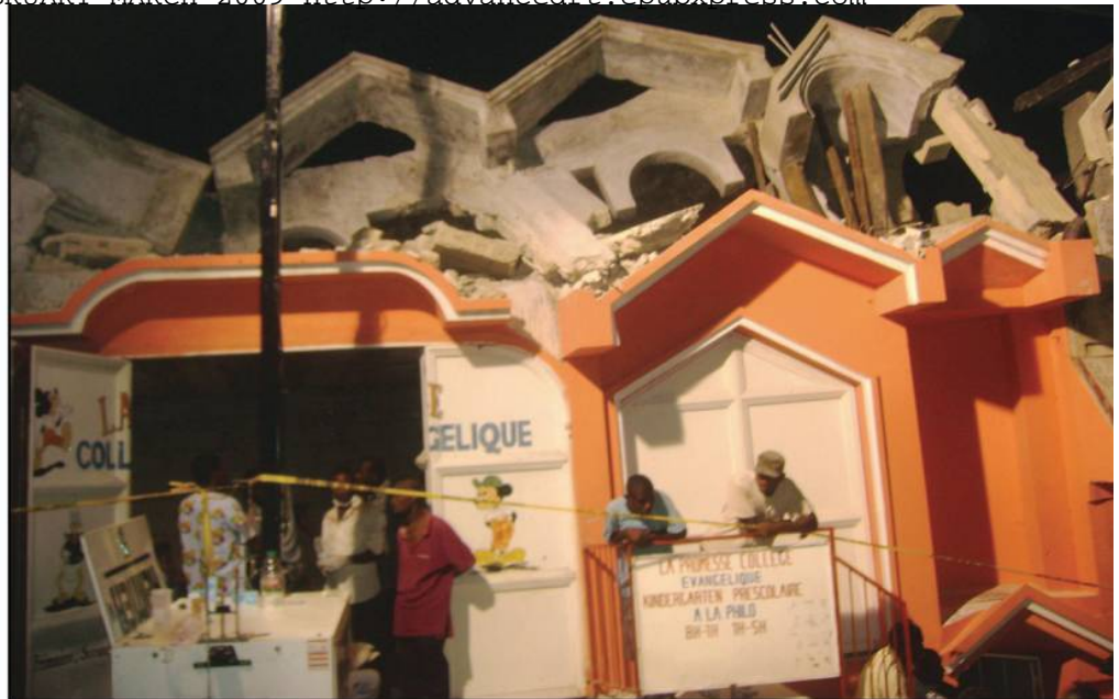
The front of the collapsed school. Photos courtesy of Nate Lasseur
